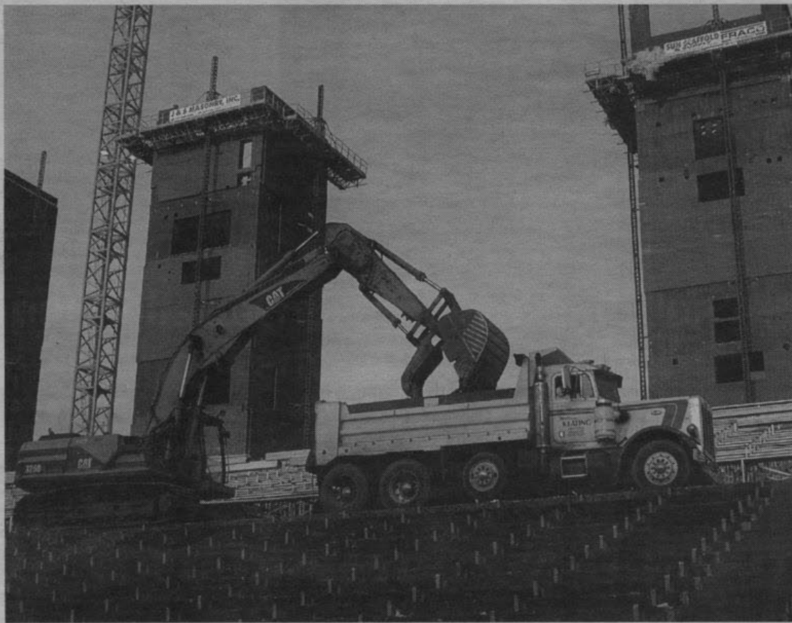
The 'Raising Reiser' project enters its next phase after the old stands are demolished following the annual Civil War game. The stadium is being expanded from roughly 35,000 to 55,000. Currently Reiser Stadium is the smallest of any NCAA Division I college in the nation. The cost for the renovations is estimated at $80 million and is scheduled to be complete before the beginning of the next football season. The renovations will add luxury boxes as well as moving Coach Mike Riley's office inside the stadium, this should help in recruitment because potential players will be able to see where they could play their college years.
