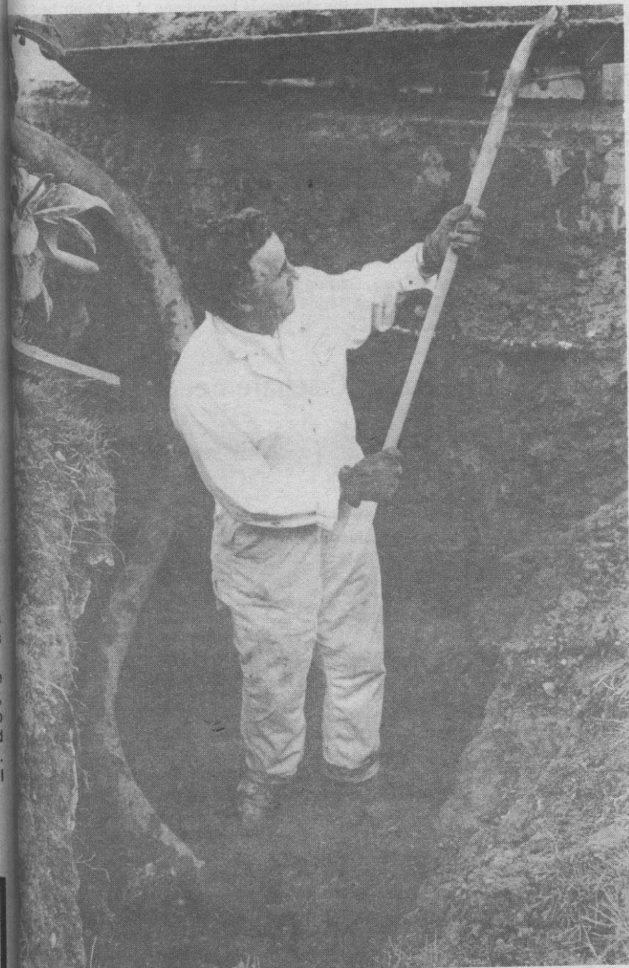
Bill you keeps the shovel moving as the grounds crew continues to hunt for a leak in water pipe. The leak was located yesterday about 3 p.m. after a full day and night of digging. The excavation took place in the LBCC quad, near the library.
