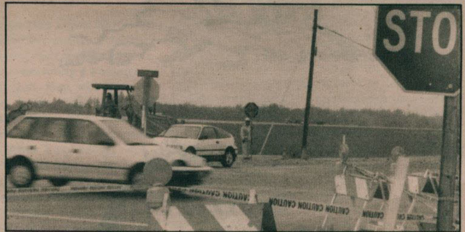
Commuters can expect slow-downs due to construction on Highway 99E. Workers will be changing the highway from a two-lane to a four-lane road.
