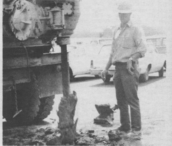
A Pacific Power and Light employee watches closely as a company machine drills a 7-foot hole for LBCC's flagpole.
